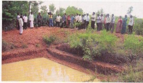
One of the ponds constructed under the project to collect rainwater at Kannanangala village in Sidlaghatta taluk in Chickballapur district.
